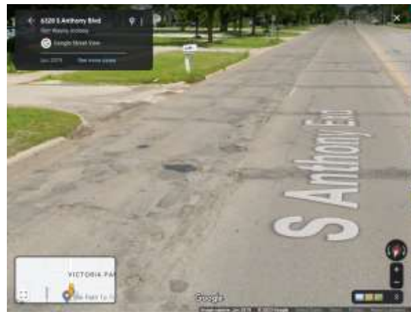
Road Surface Damage on S. Anthony Boulevard
