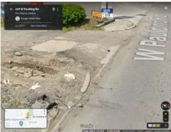
Sidewalk Damage on Paulding Road
